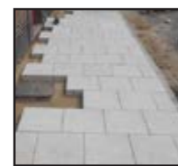
Grey Saxon paving in the process of being laid on Priory Street as a stretcher bond
